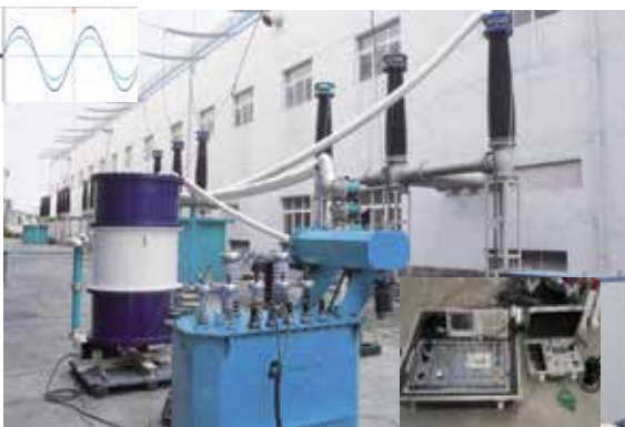
220kV GIS Synchronized AC voltage withstand on-site test in Chongqing Iron & Steel (Group) Co., Ltd
